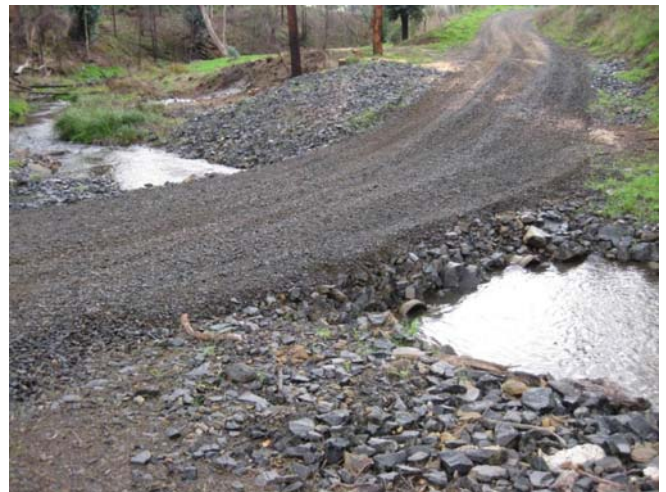
Well designed stream crossing for farm driveway or access track, Koornalla, 2010. Photographer: Penny Richards, DPI.
