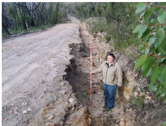
Above: Severe erosion of roadside table drain due to inadequate cross-drainage, Grampians, 2009. Photographer: Stewart Davidson, Parks Victoria.
