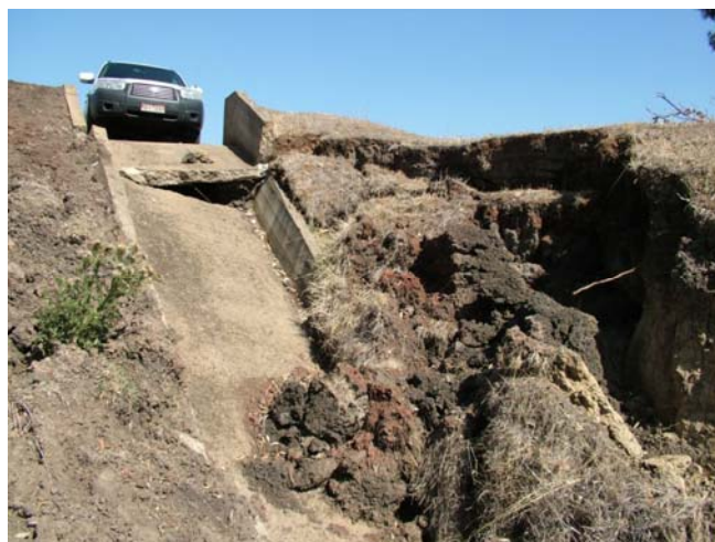
Above: Failed concrete chute in black cracking clay, Coleraine, 2008. Photographer: Clem Sturmfels, DPI.
