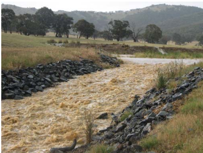
Above: Flood flows test out a newly constructed rock chute, Elmhurst, 2007. Photographer: Pauline Boatman (private collection).
