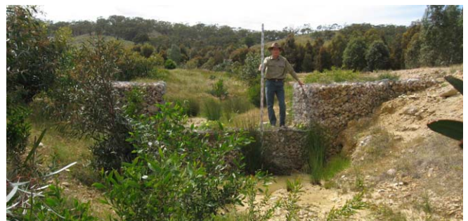
Active gully erosion stabilised with gabion weirs, gully edging and revegetation, Navarre, 2009. Photographer: Clem Sturmfels, DPI.
