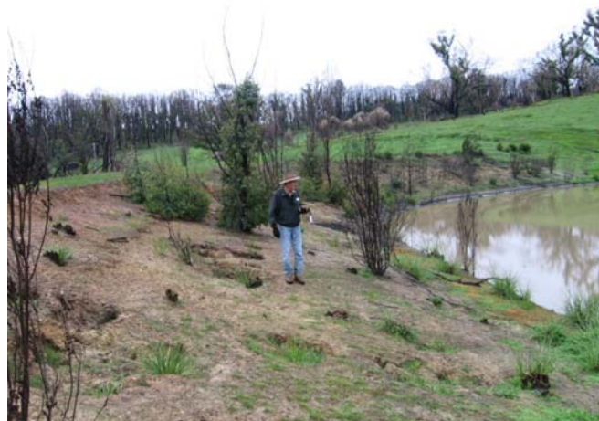
Severe tunnelling in large dam bank, St Andrews, 2009. Photographer: Tim O'Donnell, Nillumbik Shire Council.
